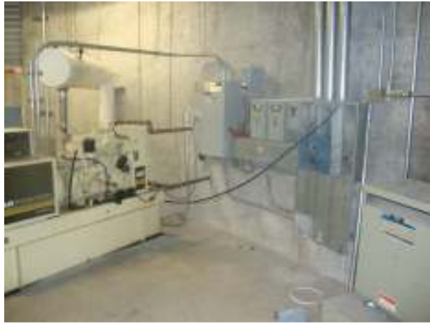
A East Electrical Room Generator, ATS, 120/208 V Transformer
