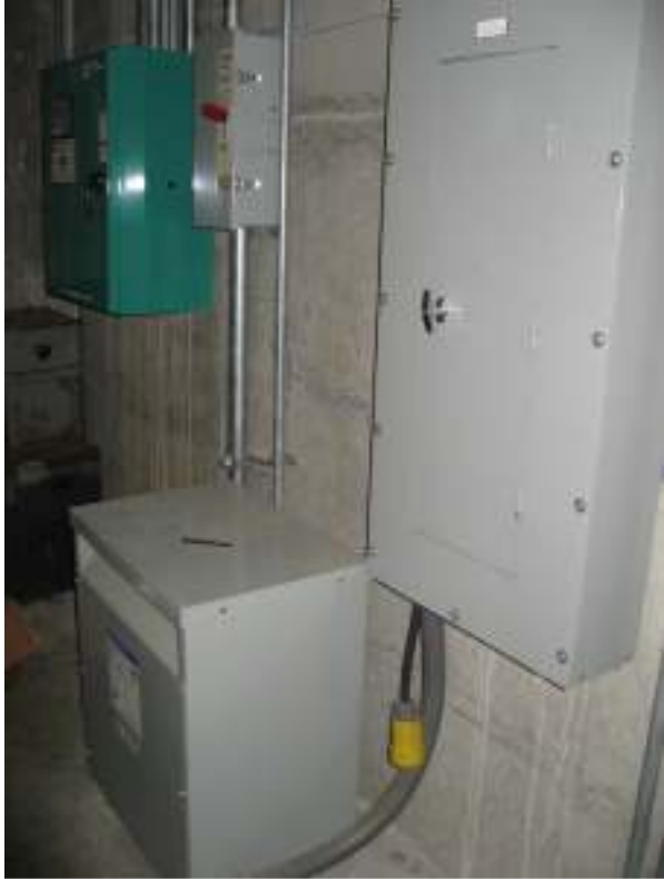
Garage E/F Normal Power Electrical Room ATS, 120/208 V Transformer & Panel EP-2B
